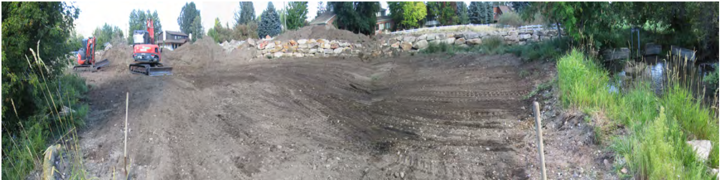
Photo 7. East view of completed fill removal in the fill removal area. Photo taken on September 15, 2023.
