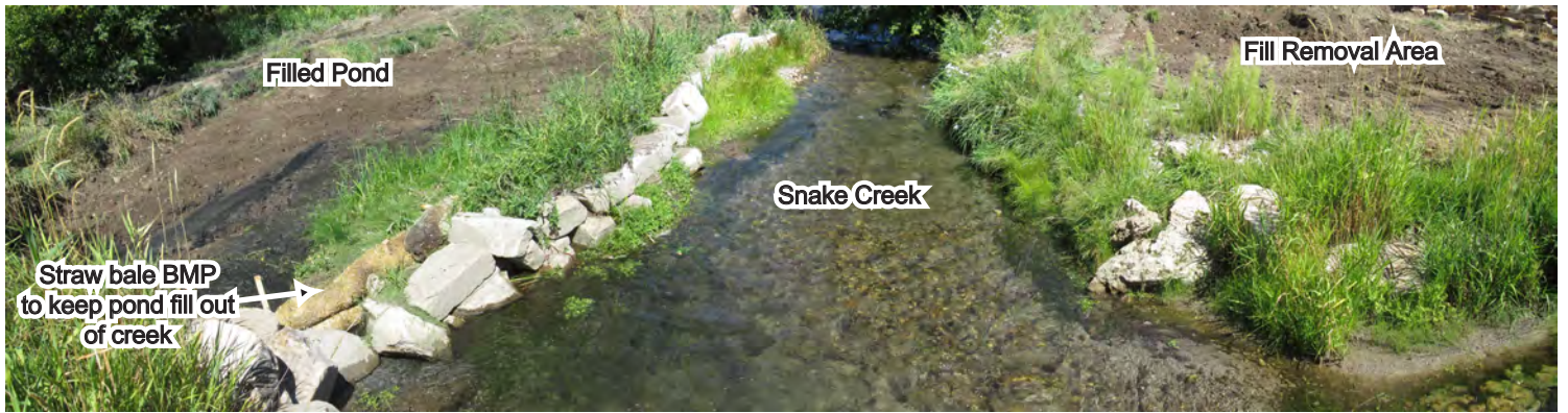
Photo 5. North view of backfilled pond (left), the straw bale BMP used to keep fill from entering Snake Creek (center), and fill removal area (right). Photo taken September 15, 2023.
