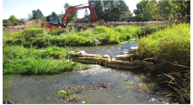
Photo 4b. South view of straw bale BMP to protect Snake Creek during back-fill of pond. Photo taken September 15, 2023.
