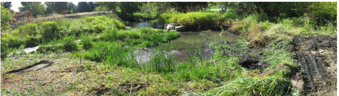
Photo 2. South view of on-going removal of the rock wall around the pond for backfilling. Photo taken September 15, 2023.
