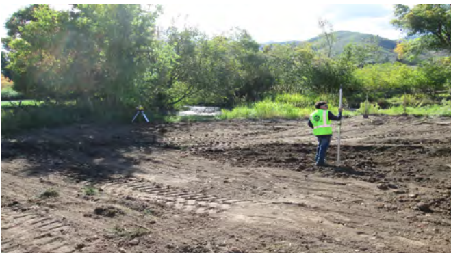
Photo 6a. Southwest view of laser-level being used to ensure proper depth of fill to remove in fill removal area. Photo taken on September 15, 2023.
