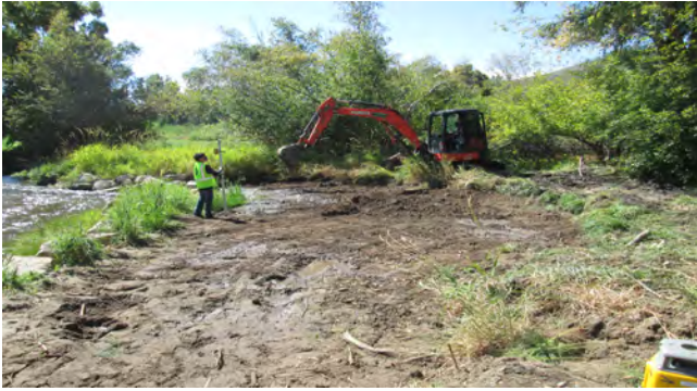
Photo 4a. South view of pond backfill being leveled using a laser-level. Photo taken September 15, 2023.
